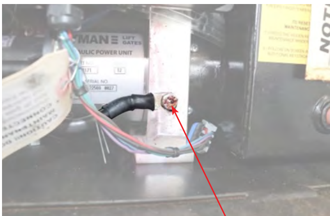
Ground to Side of Power Unit
