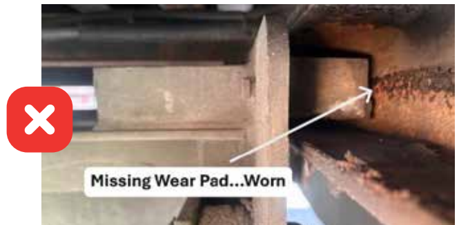
Bad Skid Wear Pad Adjustment
